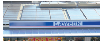
Solar panels with a 22 kW* power-generation capacity at the Kodaira Tenjincho 2-chome store
