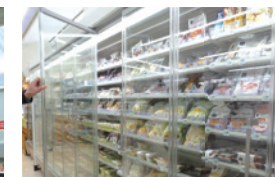
Double-pane glass enclosing the cold cases significantly limits leakage of cooled air.
