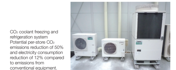
CO 2 coolant freezing and refrigeration system. Potential per-store CO 2 emissions reduction of 50% and electricity consumption reduction of 12% compared to emissions from conventional equipment.
