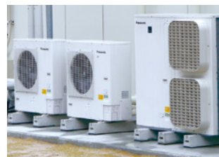
CO 2 refrigerant cooling/refrigeration system
