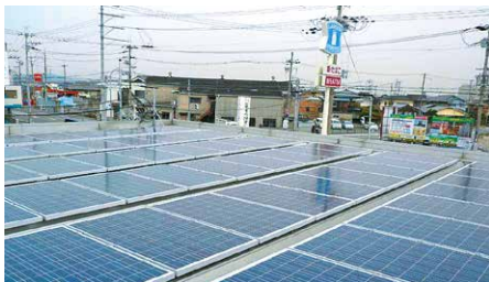
Installed solar power generation equipment on the roofs of approximately 2,000 stores. Further strengthening renewable energy introduction
