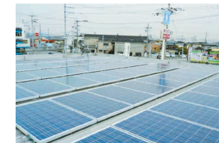
Solar power generation systems
