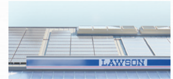
Solar panels equivalent to 22 kW installed at the Kodaira Tenjin-cho 2-chome Store (exceeding the usual 12 kW)
