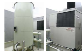
Biomass power generators
