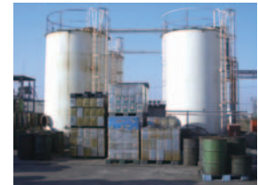
▶ Waste oil recycling plant
