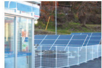
▲ Solar power system
