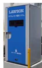
Lithium-ion battery system
