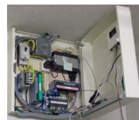
The advanced automatic energy monitoring and control system
