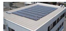
Solar power system
