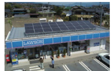
▲ Solar power generation systems using citizen funds
