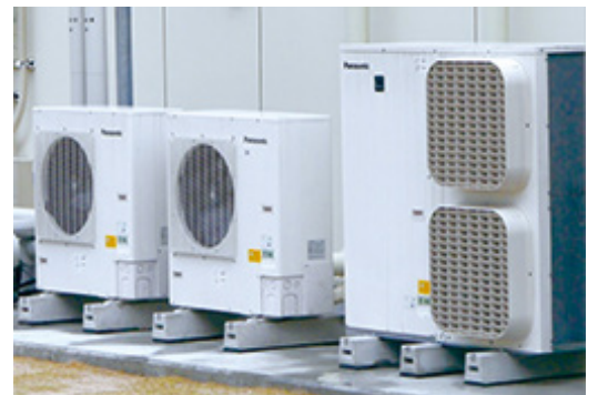
▲ CO 2 coolant freezing and refrigeration system
