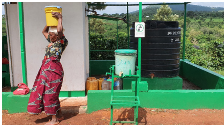
Water tank installed at the AVIV Farm
