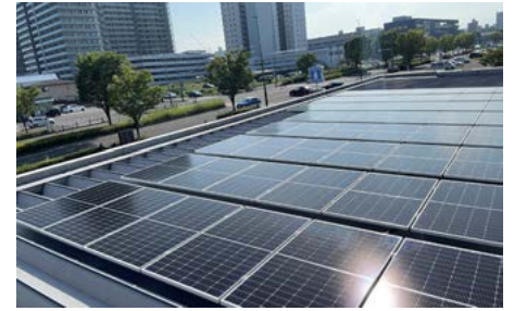
▲ Solar power generation systems
